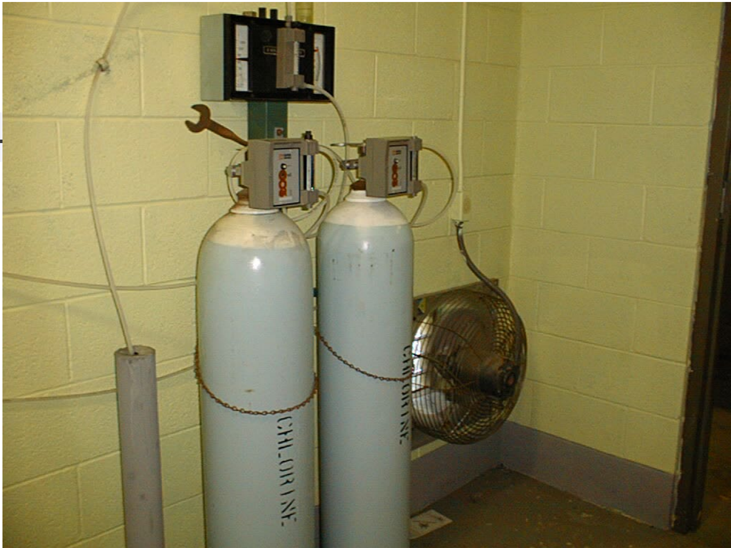
Cylinders chained down, wrench on shutoff, exhaust fan near the floor.
